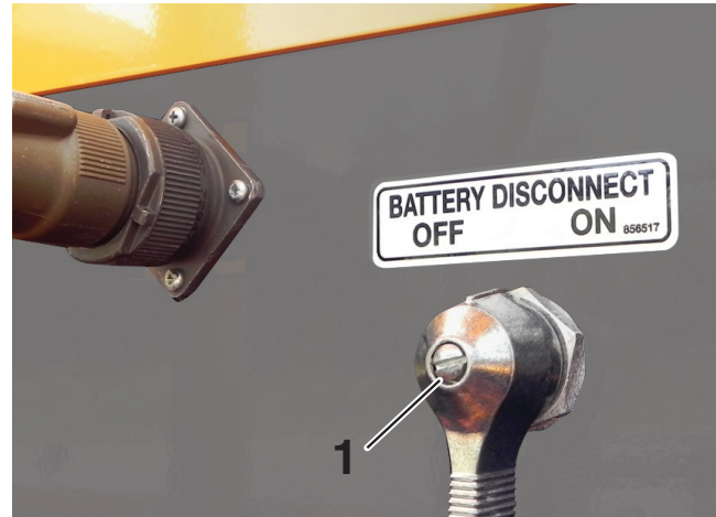
Battery Disconnect Switch
