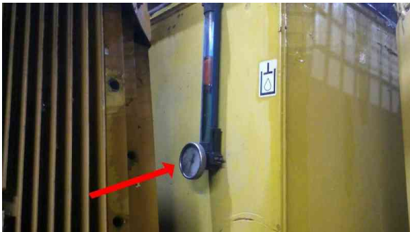
Gauge not working, have to be replace
