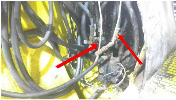
Cut wires under the operator console
