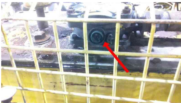
Filters gauge broken, need to be replaced
