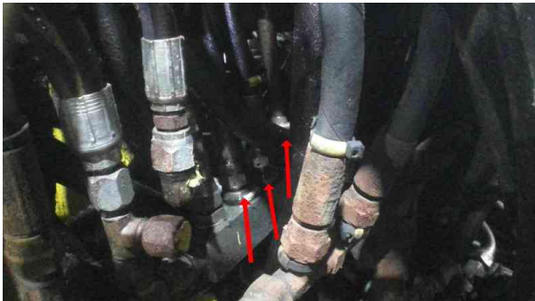
Leak under the operator console
