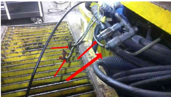
Brake sensors broken, need to be replace
